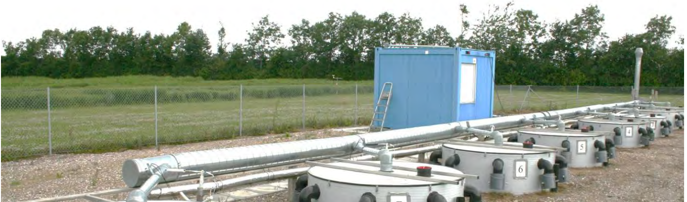
Pilot-scale storage facility used in this study.
